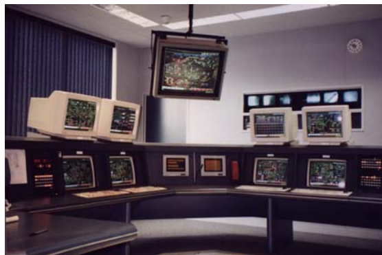
UNISON® Control Room
