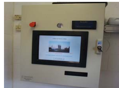
Self - Service Loading Kiosk
