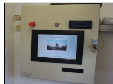
Self - Service Loading Kiosk
